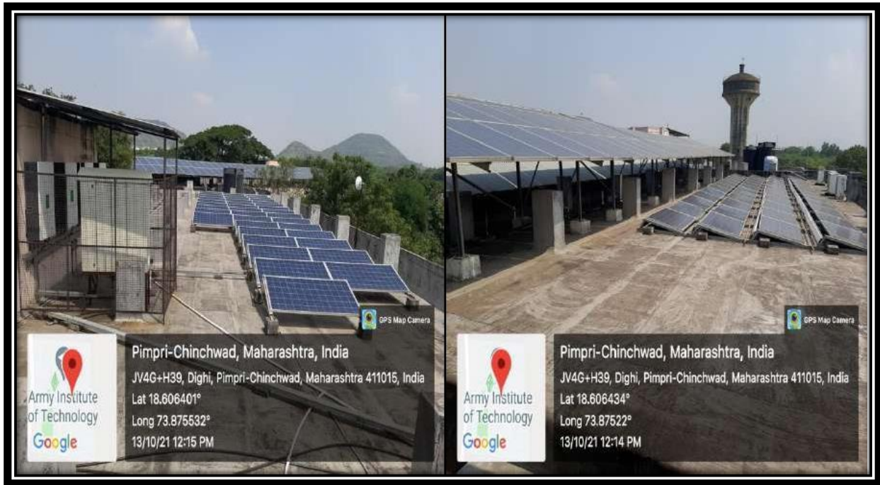
Rooftop Solar Panel
