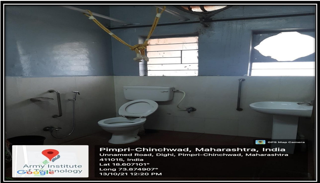
Disabled Friendly Washroom
