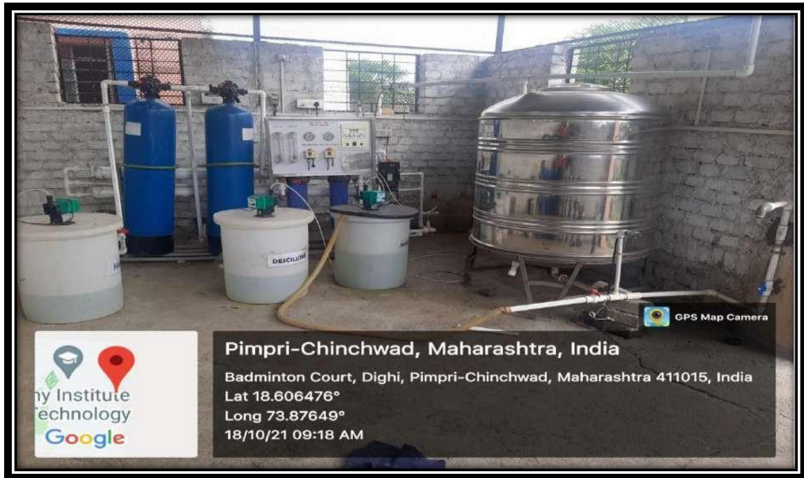
RO Water Plant
