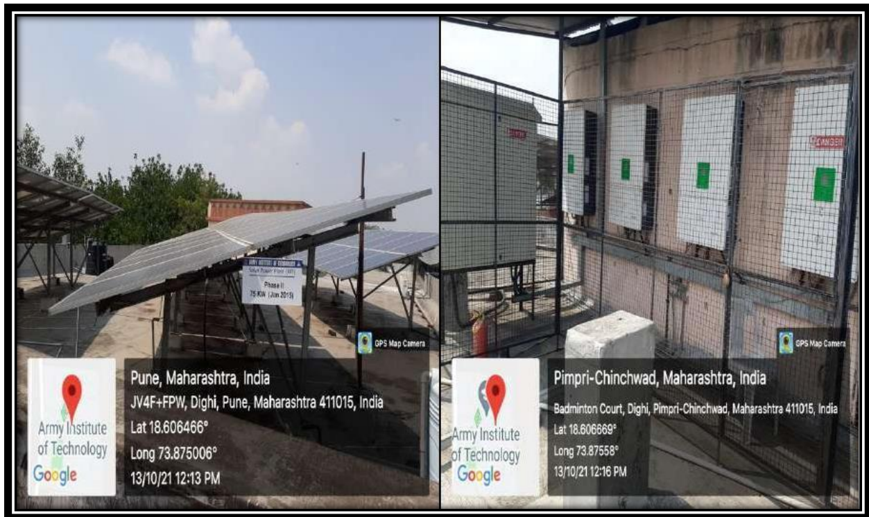
Rooftop Solar Panel
