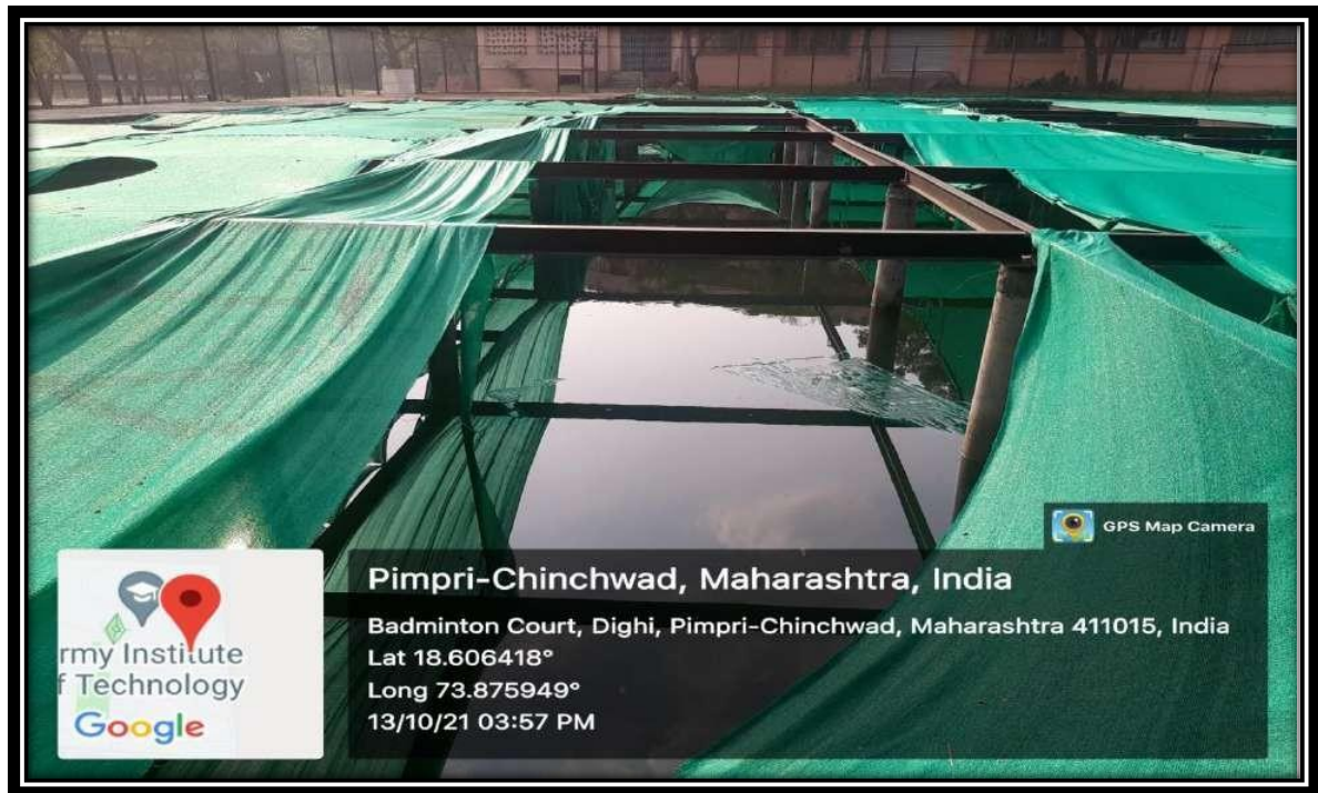
Rain Water Storage Tank
